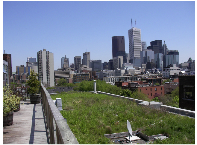
Fig. 5. Green roof on 215 Spadina (meadow-like green roof with physical access).
