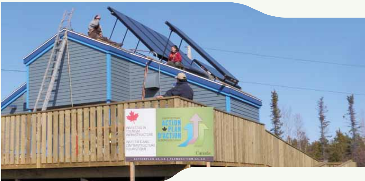
The Fred Henne solar hot water installation.
