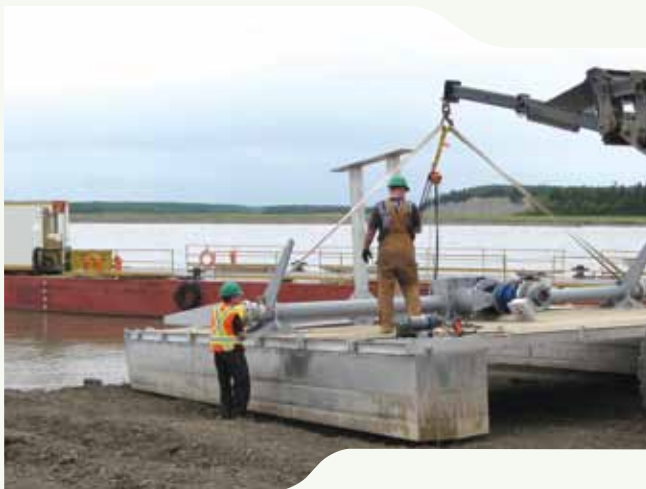
Assembling and preparing to install the hydrokinetic turbine in the Mackenzie River at Fort Simpson.
