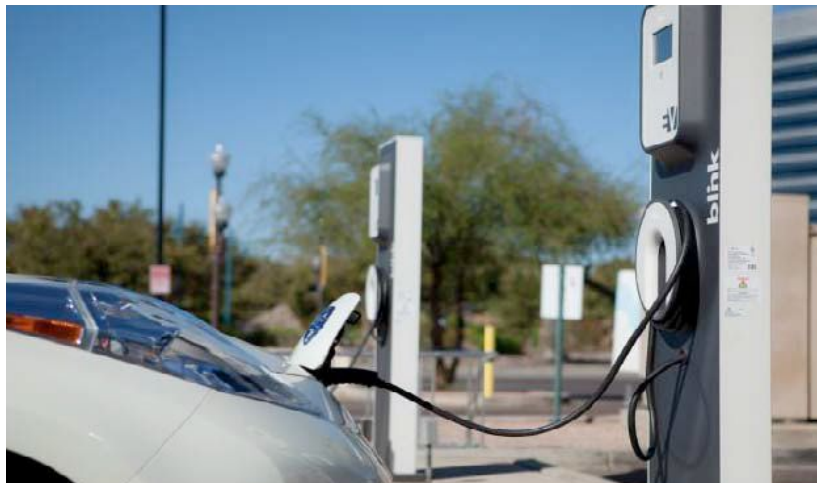
Fig. 8: Level 2 charging station
