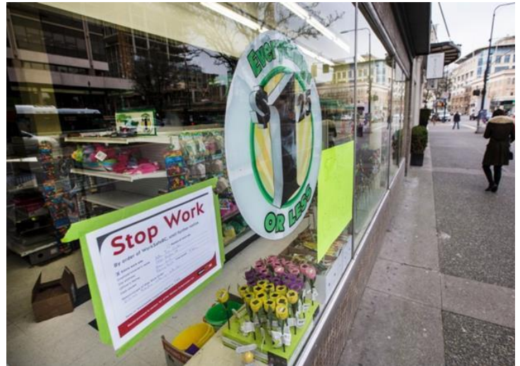
The Dollar Tree store in downtown Victoria has been closed by WorkSafeBC prevention field officers because of concern that crumbling floor tiles containing asbestos could cause harm (The building assessed to worth $1.7 million). Adopted from Times Colonist 2017-03-01.
