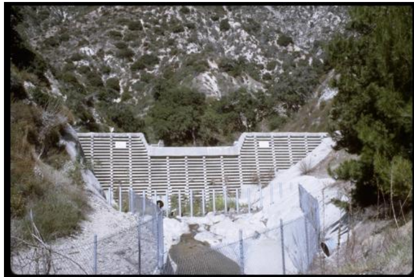
Figure 4: Debris flow catchment structure which stops large solids from passing, but allows water and fine sediment to travel downstream.
