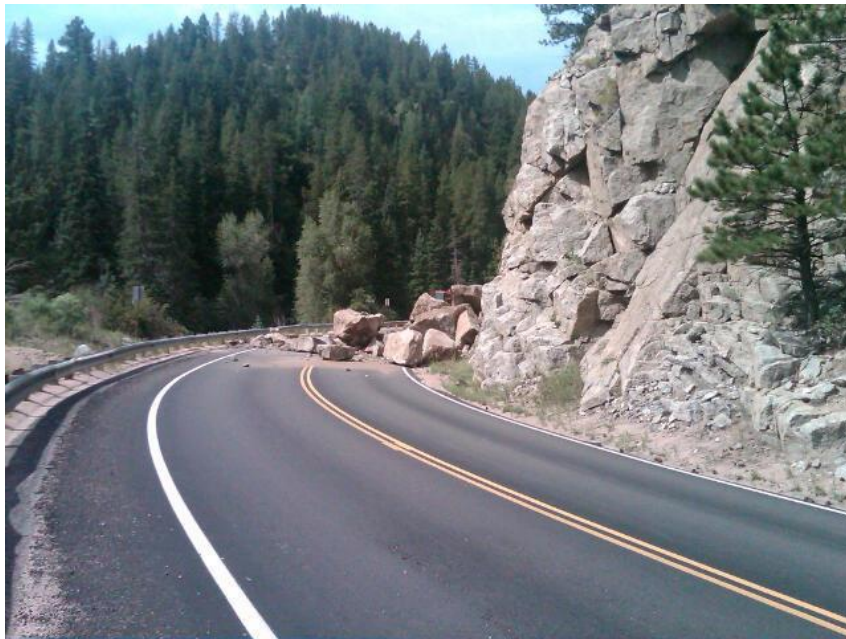
Figure 2: Rock fall from a steep roadcut.
