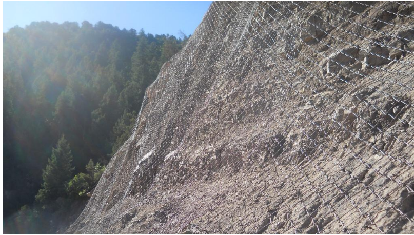
Figure 3: Rock fall netting used to capture large chunks of rock, and allowing them to pass safely to the base of the net.
