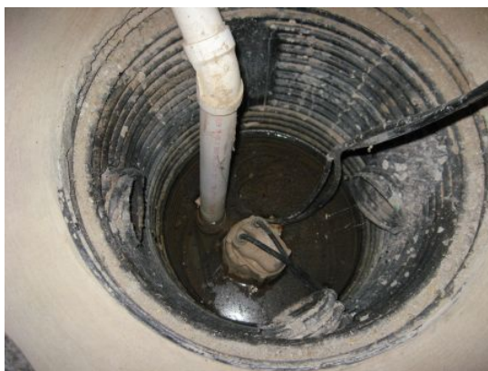
Figure 6.17: A sump crock.
